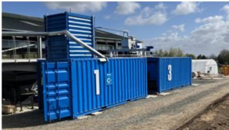
The Containerised Combined Heat and Power (CHP) and AD system from Organic Power Ireland.
