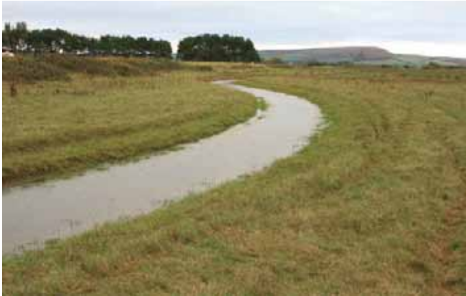
Recreating a meandering stream where only recently, there was a canalised ditch.
